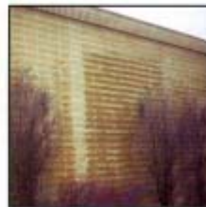
New concrete block wall showing water retention after a rainstorm.
