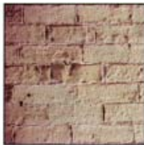
Heavily eroded brick resulting from sandblast abrasion.
