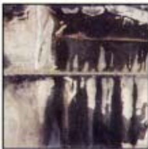
Typical pollution dirt crust showing stone surface flaking.
